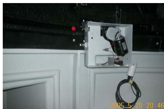
Dome Rotation Motor Box
